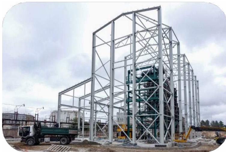
Ventspils recovery plant during construction process. Courtesy of PSIA Ventspils labiekārtošanas kombināts
